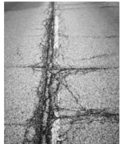
▲ Pavement ravel and erodes along open cracks causing deterioration.
