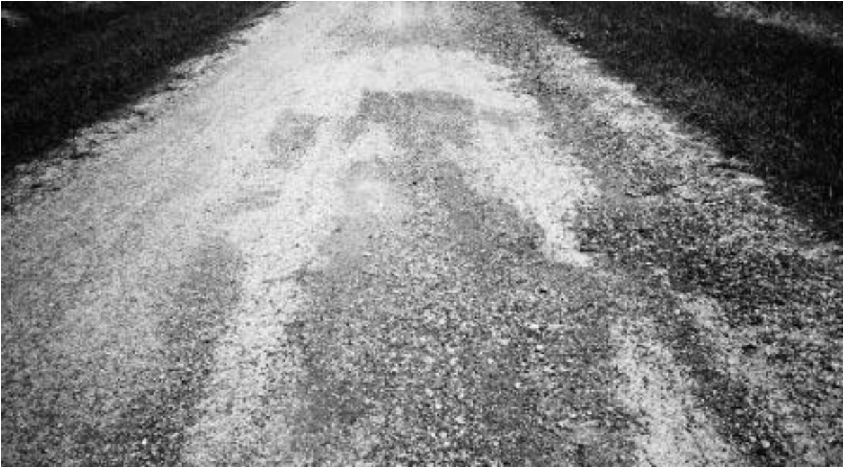
◀ Extensive loss of surface. Rebuild.
