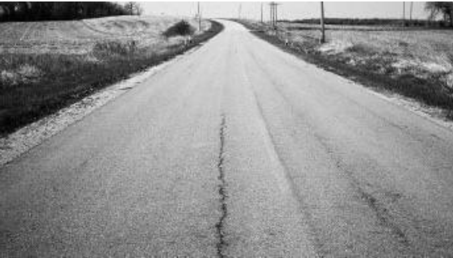
◀ Longitudinal cracking; early load-related distress in wheel path. Strengthening needed.
