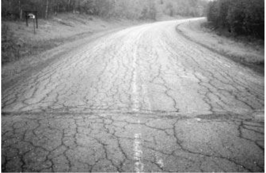
▶ Extensive alligator cracking. Pulverize and rebuild.
