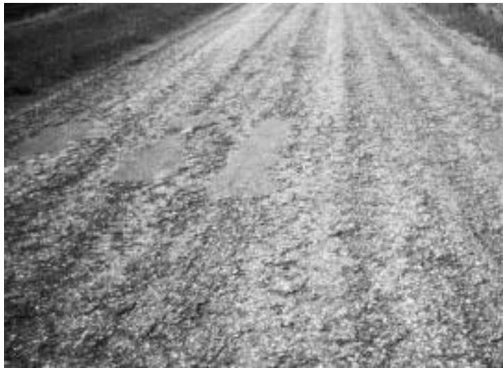
◀ Severe raveling and loss of surface material.
