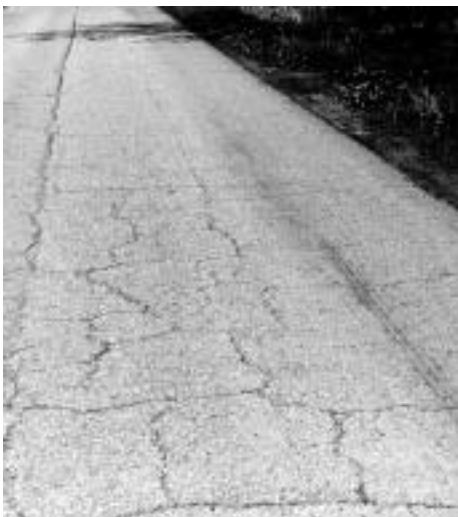
▲ Extensive block cracking in an irregular pattern.
