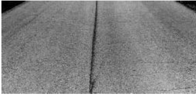
Centerline crack (still tight). ▶
