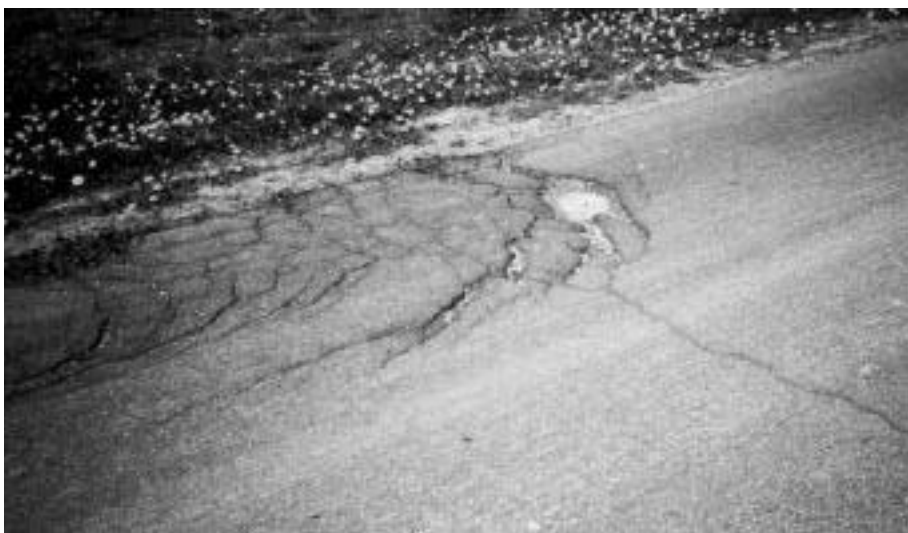
► Crescent-shaped cracks characteristic of slippage.
