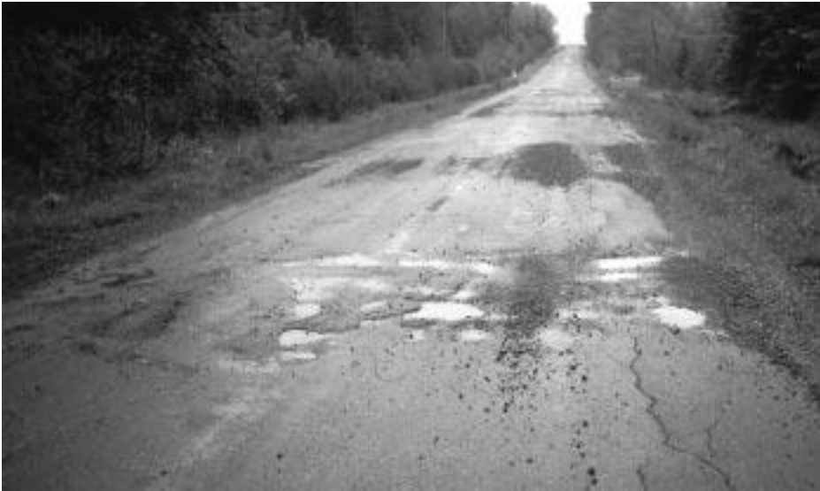
◀ Potholes from frost damage. Reconstruct.
