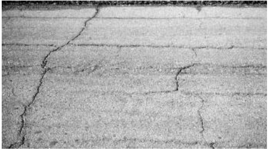
▼ Block cracking with open cracks.
