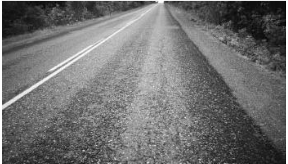
► Moderate to severe raveling in wheel paths.
