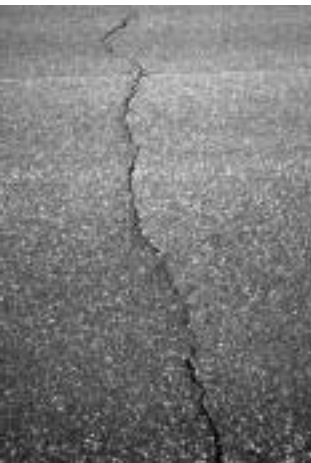
▲ Tight cracks less than 1/4" in width.
