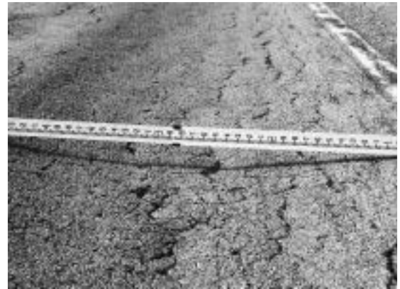
▲ Severe rutting. Strengthen base and reconstruct.
