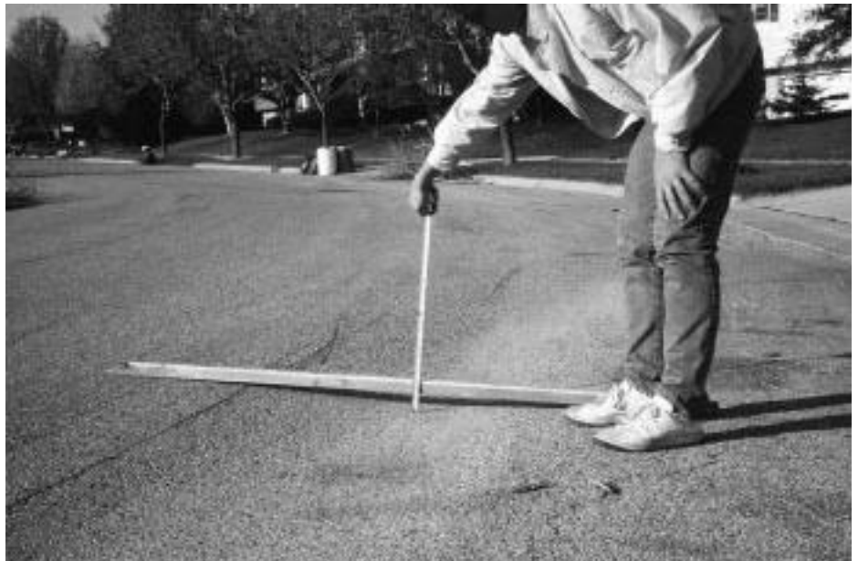
► Severe settling from utility trench.
