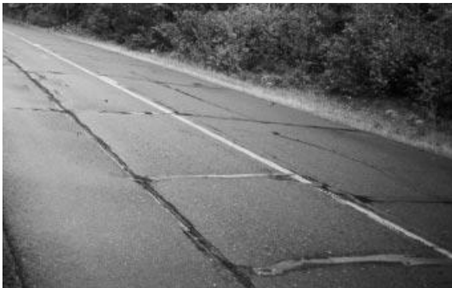
► Concrete joints reflected through bituminous overlay.
