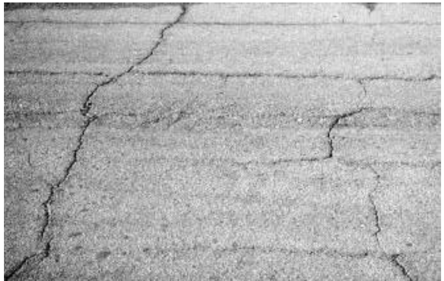
▶ Intermediate-size block cracking, 1'-5' across with open cracks.
