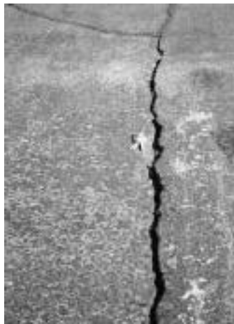
▲ Open crack – 1/2" or more in width.
