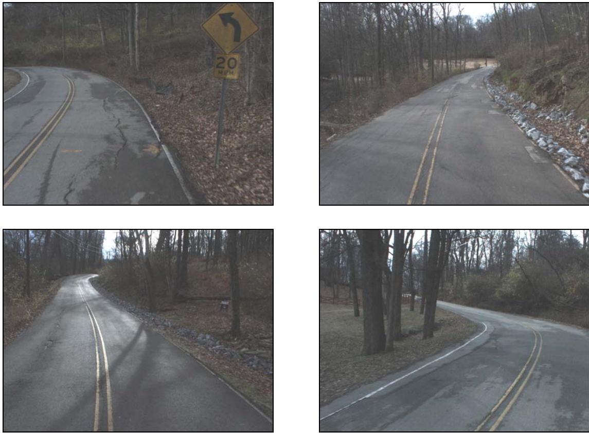
Figure 1: Existing Pavement Distresses
