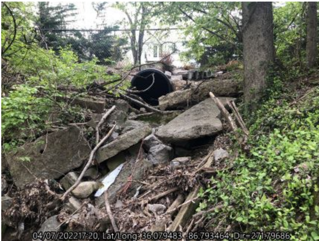
Photograph 6: Watercourse 1 in the upper portion of the reach with concrete slabs and a drain opening at the head of the watercourse.
